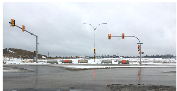
Roadway under construction to connect Rosewood residential area to Meadows Market on the east side of the Rosewood Neighbourhood
